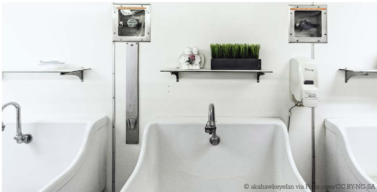
Figure 3.2.2. An emergency wash stations.
