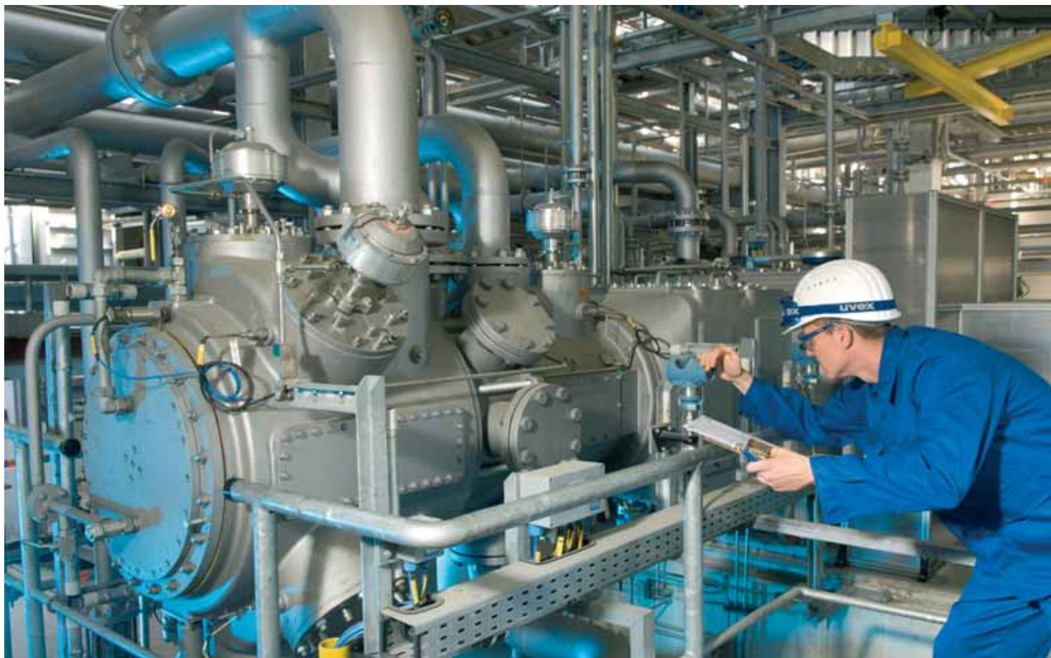
Maintenance work being conducted at the recycle gas compressor at the Sasol O&S plant in Brunsbüttel, Germany.
